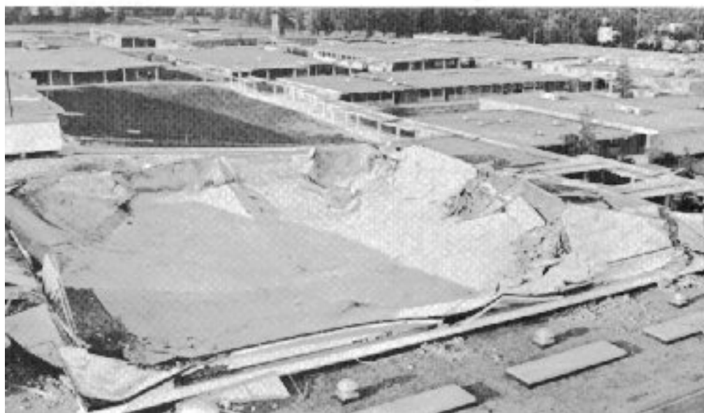
Figure 1. Newspaper photograph of the collapsed hypar shell [1]
